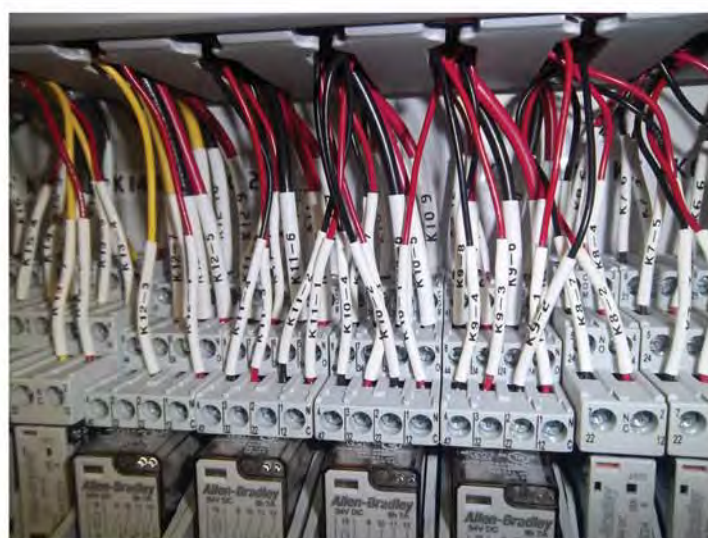
Close-Up of relay section showing every wire labeled
