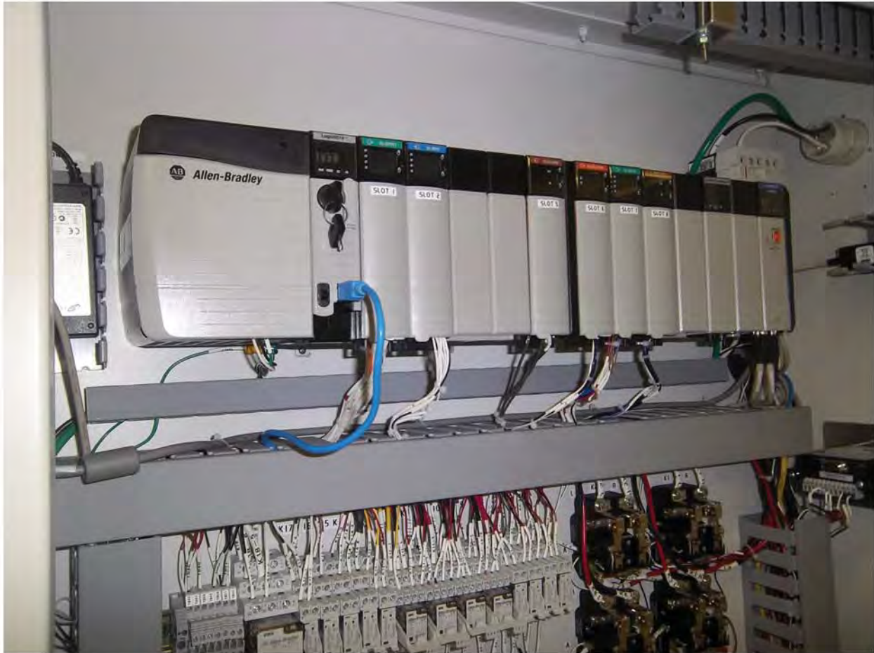
Close-Up of Programmable Automation Controller used to control the System
